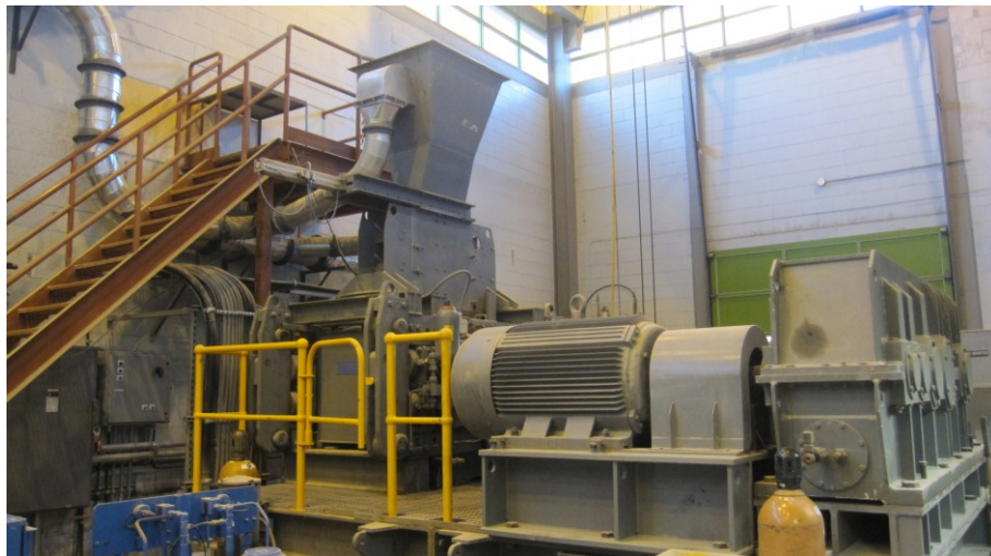
Figure 3.9 Pilot HPGR installed at UBC
