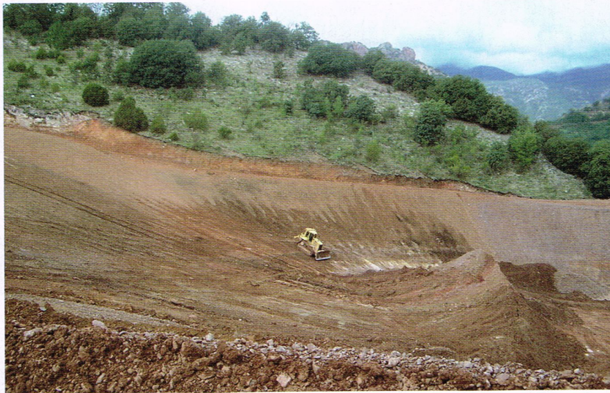
Building the leach pad in 2007 at Minefinders' Dolores gold mine in Sonora, Mexico.
