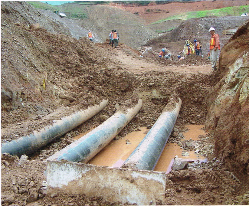
Pipe penetrating the buttress at Minefinders' Dolores gold mine in Sonora, Mexico, circa 2007.
