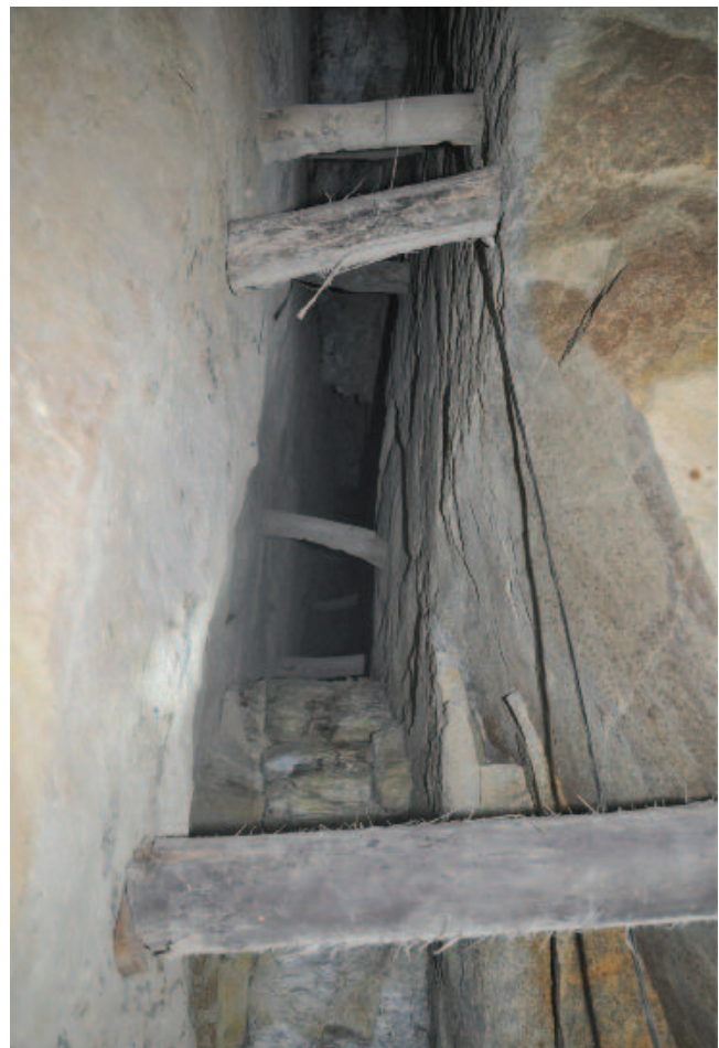
Figure 14: Narrow-vein open stoping, using timber props as support. Chollja, Bolivia. Vein zone is less than 1m wide.
