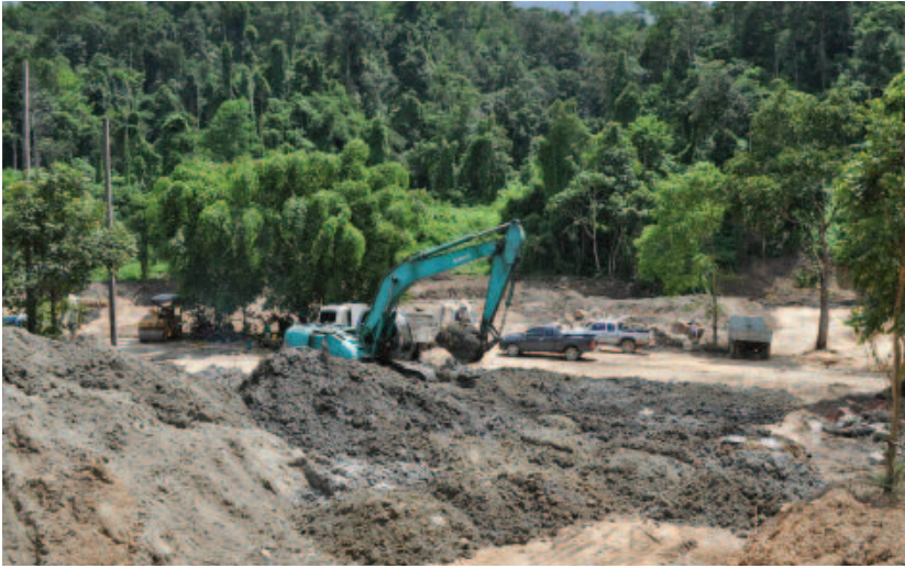
Figure 52: Tailings Retreatment: Rehandling and homogenisation of tailings at the historic Sritorranee mine near Chiang Mai ahead of transport to the flotation plant at Lampang Mineral and Metal (Thailand) Ltd.
