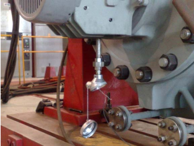
Figure 2. RTD for Bearing Oil Sump Temp. Measurement
