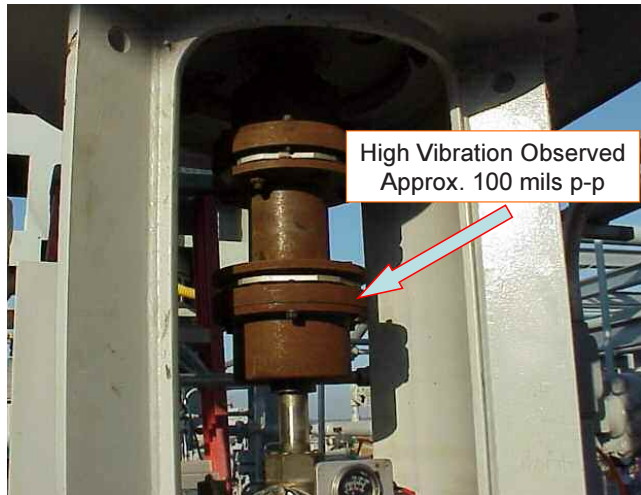
Figure 7. Excessive Vibration on Pump Coupling and Pump Shaft.
