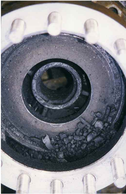
Figure 15. Impeller from Pump A During Disassembly after Pump Failure. (Note carbon particles and dust from destroyed carbon bushings.)
