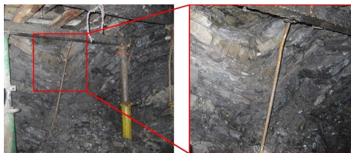
Figure 3. Caving roof near the working face end.
