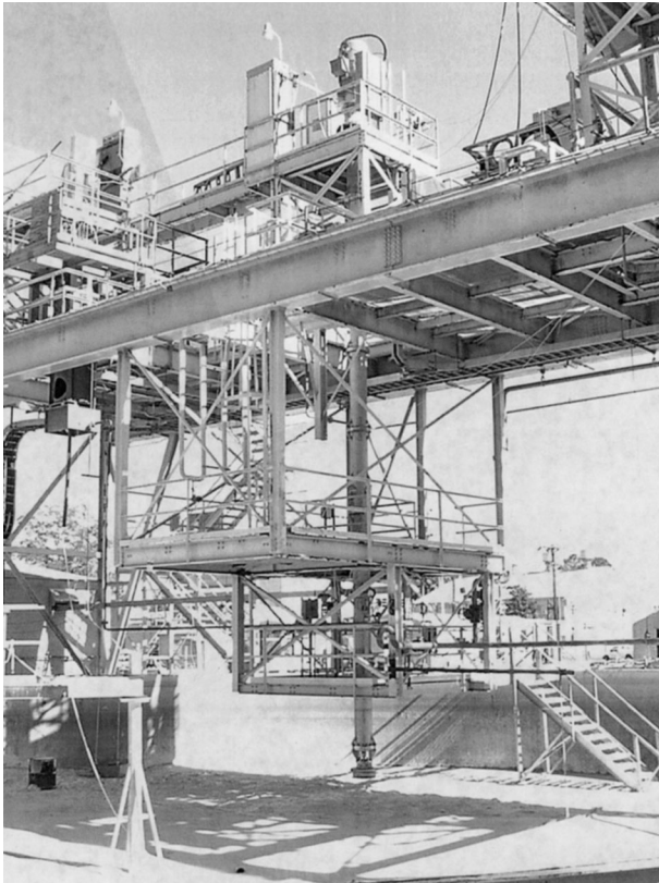
Figure 6. Pump Installed in Vibration Test Facility.
