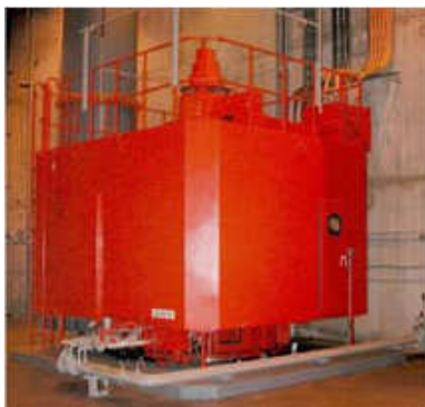
Figure 10. Wastewater treatment vertical mounted motor (Courtesy of TMEIC)
