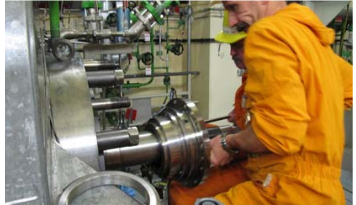
Figure 12: Installation of the first seal with Diamond Face® technology in a reactor feed pump at the Nuclear Power Station Isar I
