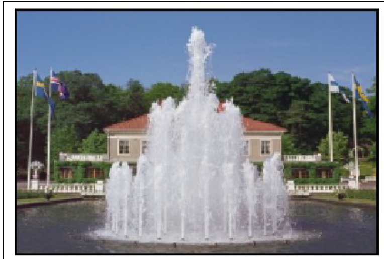
Fountain pump system
