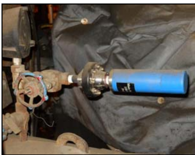
Figure 3. Tee Connection with Local Pressure Gauge (Vertical- Left) and Wireless Pressure Sensor with Battery Powered Transmitter (Horizontal-Blue).
