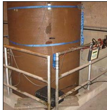
Figure 12. Ultrasonic Flow Meter with 4-20mA Transmitter and Signal Repeater (Black Box).
