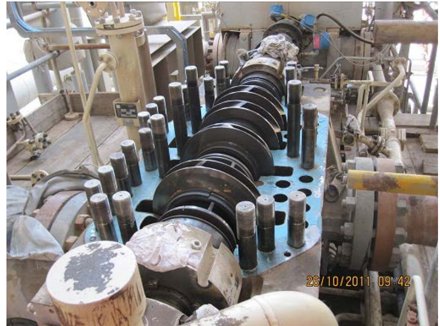
Old pump at skid in RGX2
