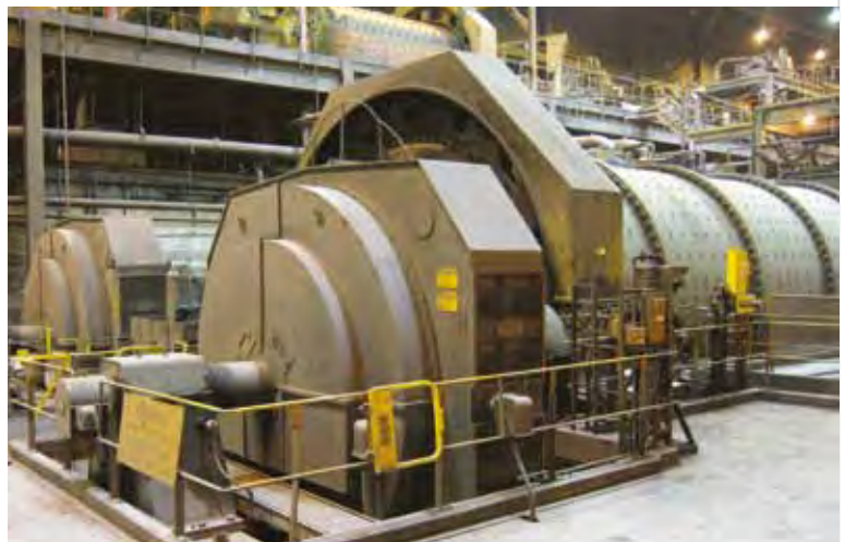
Synchronous motors 3000 HP at 164 RPM with DPG enclosures driving a dual pinion ball mill at an iron ore mine.
