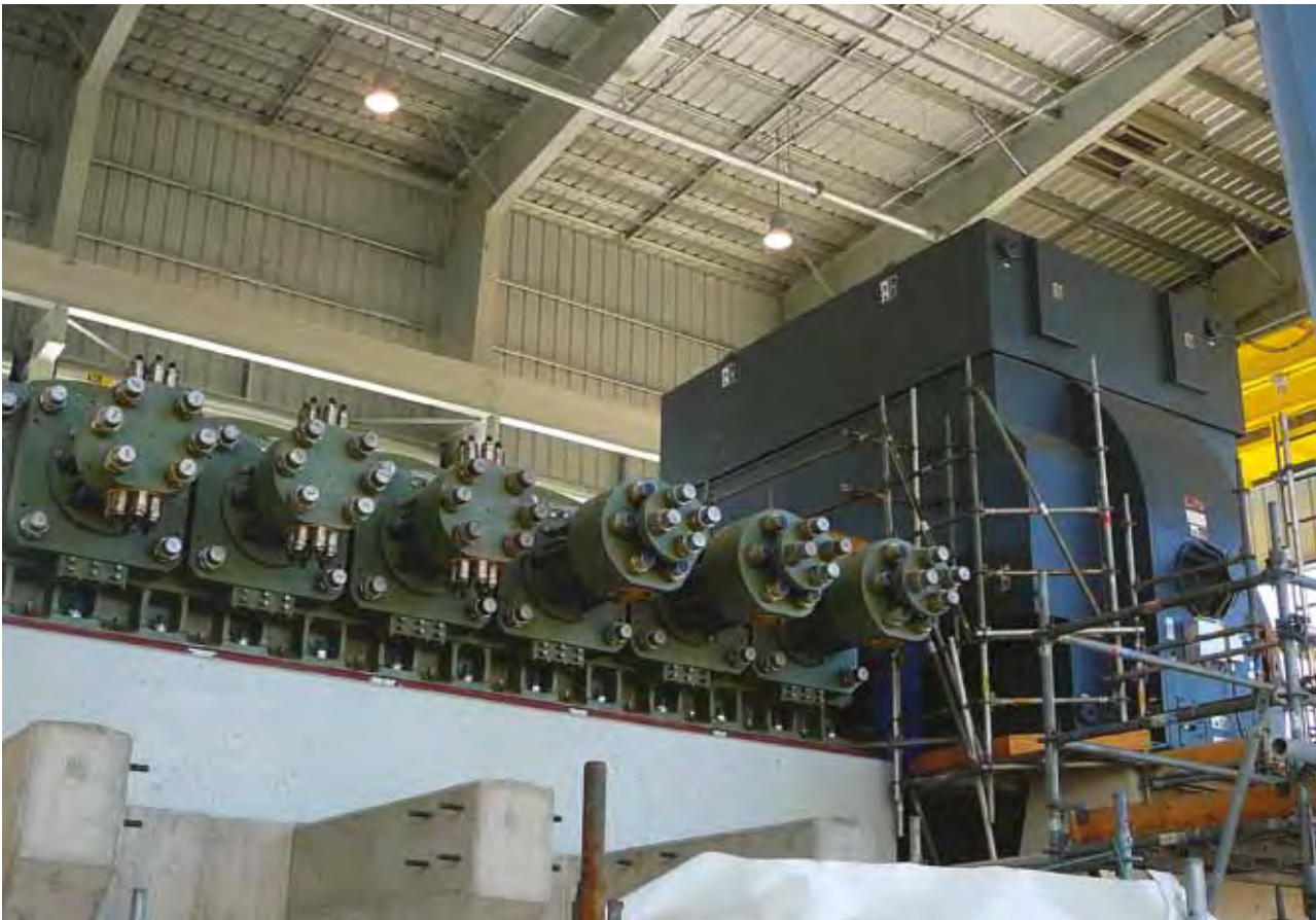
Synchronous motor 24800 HP at 225 RPM with TEWAC enclosure driving a reciprocating compressor at a polyethylene plant.
