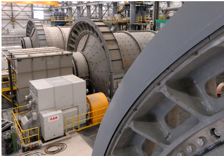
Figure 7 – ABB synchronous motor on Ball Mill 1
