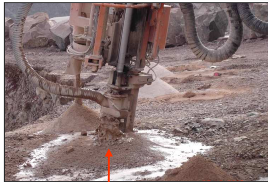
Burst of inhole water
