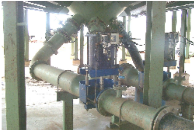
Cone and Pinch Valve Arrangement
