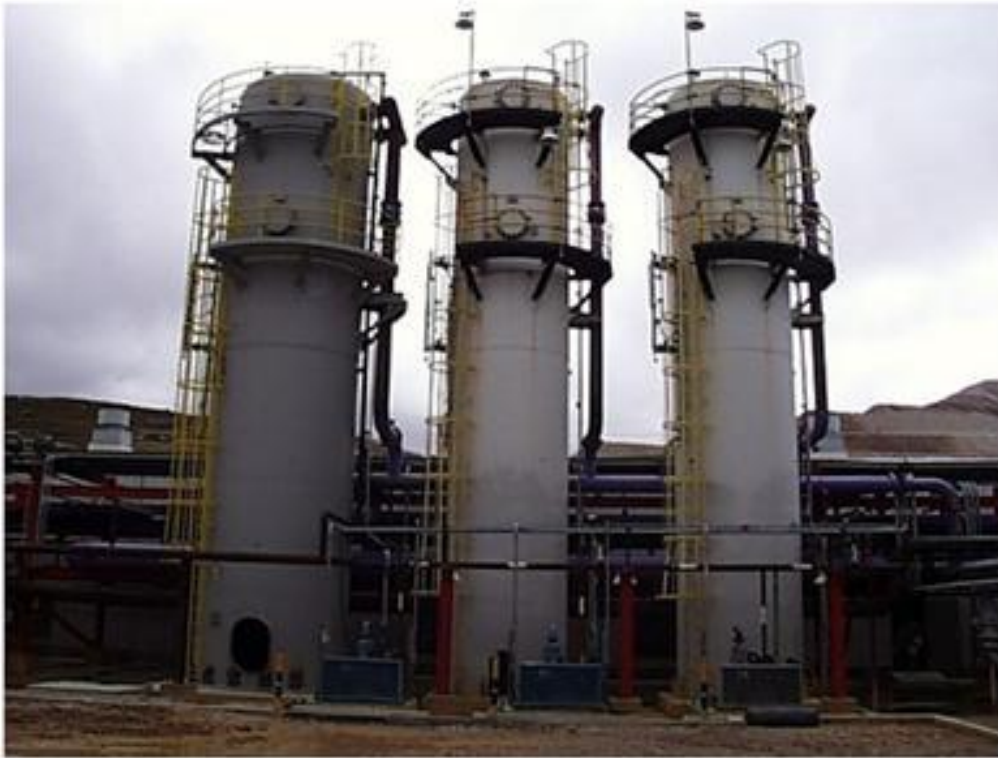
Figure 8: A picture showing three de-aeration towers
